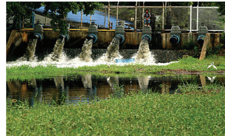
Partially treated wastewater flows into constructed wetlands for final treatment
